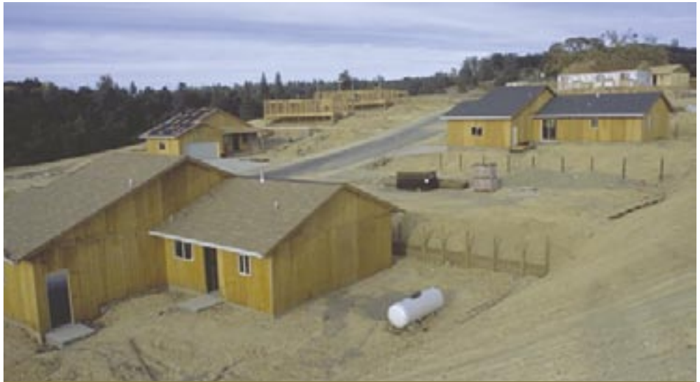
These homes in Placerville, CA are being built through USDA's self help program.
