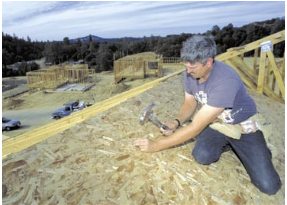
Bill Adkisson works on the roof of the Placerville, CA home he's building in conjunction with USDA's self-help program.
