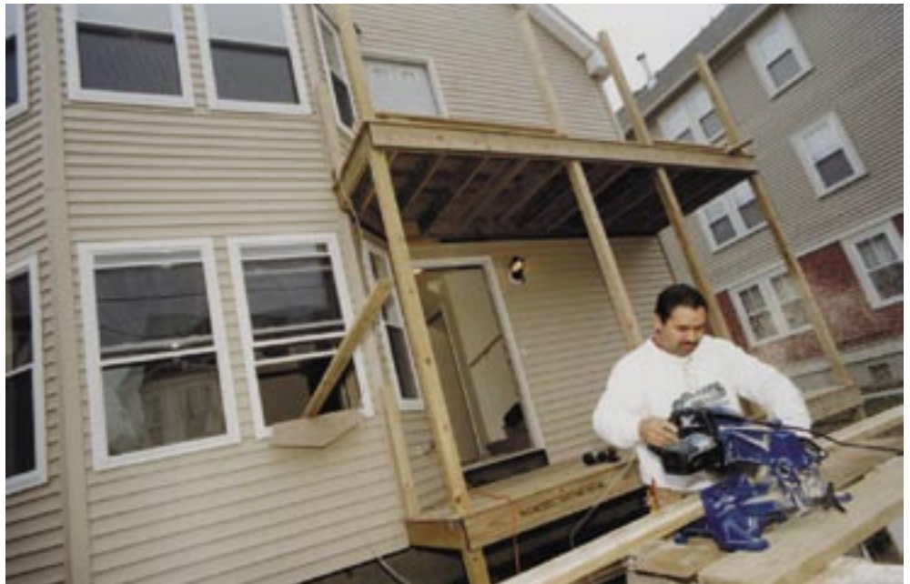
Jose Santiago repairing a porch in conjunction with a NeighborWorks® initiative in Providence.
