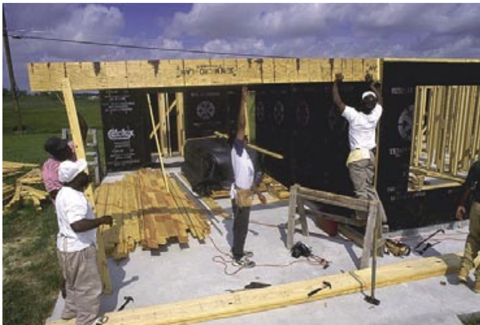
“Self-help” workers put a support beam into place at one of the self-help homes under construction in Indianola, MS.
